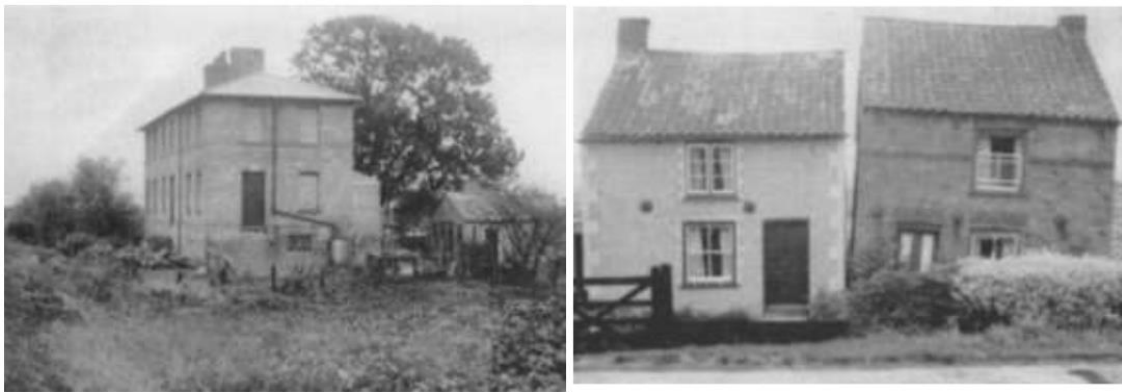
Figure 3-1 Examples of peat subsidence affecting buildings (taken from Susan Page et al. 2020; originally from Thompson 1957).
