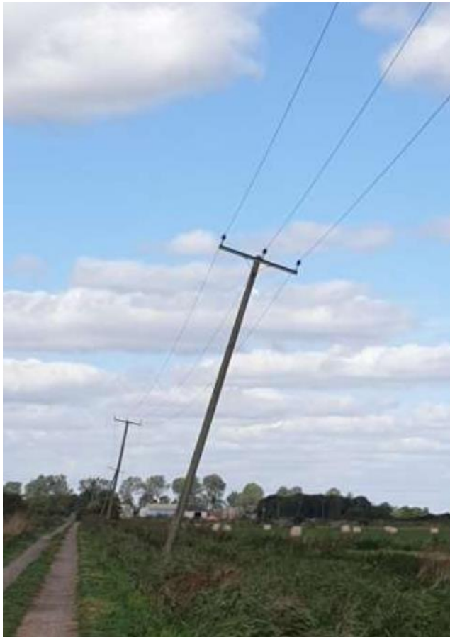
Figure 3-2 Pylons affected by peat subsidence (Photo: Sue Page, taken from Page et al., 2020).
